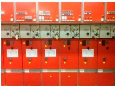
Portholes placed on Alstom cells.
