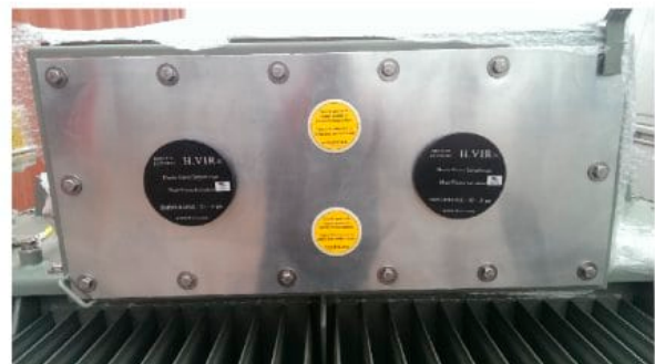
H.VIR 85 on oil transformer.
