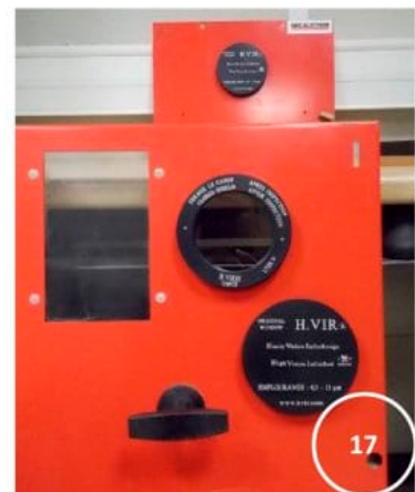
Electrical equipment ready for inspection.
