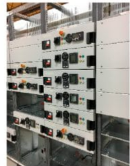
H.VIR implanted on LV switchboards.
